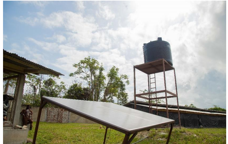
Solar panel and water pump
